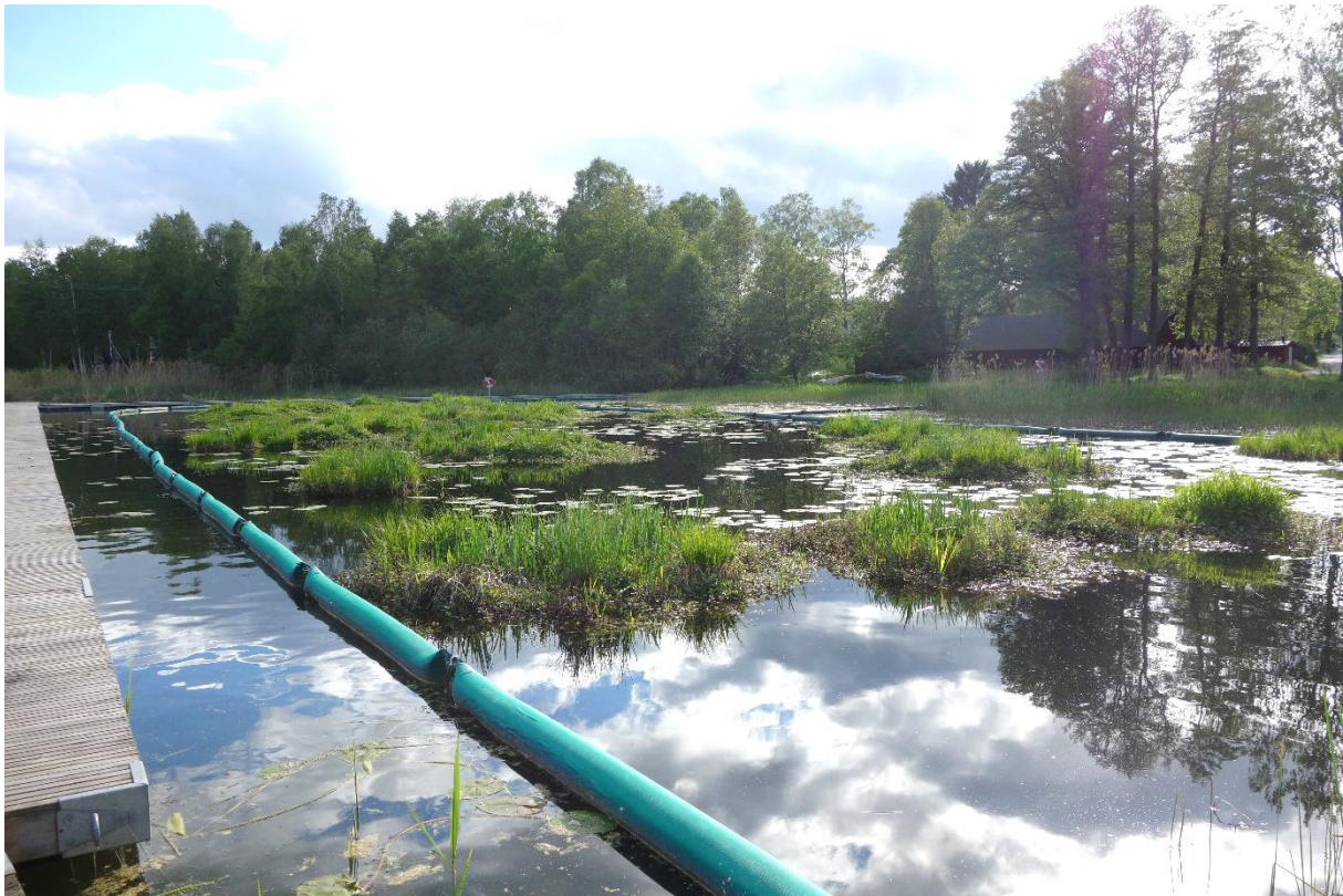
Fig 2. Floating treatment wetland installation inside floating baffles in Rönningesjön, Täby outside Stockholm. Stormwater with increased levels of phosphorous passes the FTWs before it is released into the lake.
