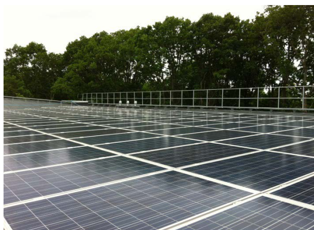
Figure 2: Photovoltaics installed on the roof of the retirement home in the passive house area Vallda Heberg [6].
