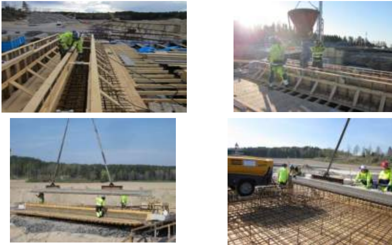
Figure 17: Construction steps for Group IV: a) Formwork, b) Concrete pour, c) Lifting to the bridge deck slab, d) Final position before casting of the bridge deck
