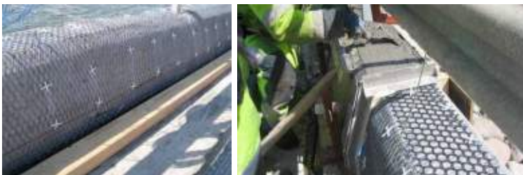
Figure 11: a) Installation of cathodic net and b) concrete cast in the edge beams of the bridge in Öland (Maglica, 2012).
