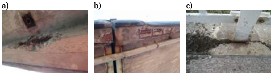
Figure 10: Critical locations of the BEBS: a) Drainage, b) Expansion joints, c) Railing post
