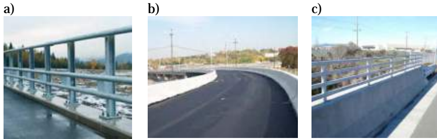
Figure 6: BEBS with different railing types: a) steel, b) concrete and c) mixed
