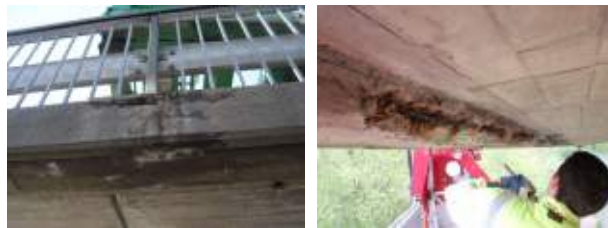
Figure 1: Examples of deteriorated BEBS in the need of LCMs to be carried out
