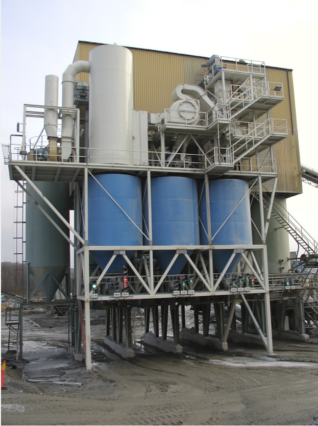
Buell-installation hos NCC Roads Stenungsund.
