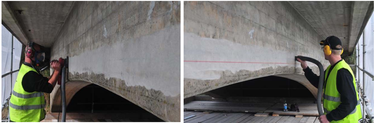
Fig. 5.2 Preparation of the concrete surface by grinding (left) and removing the dust from the ground surface (right).
