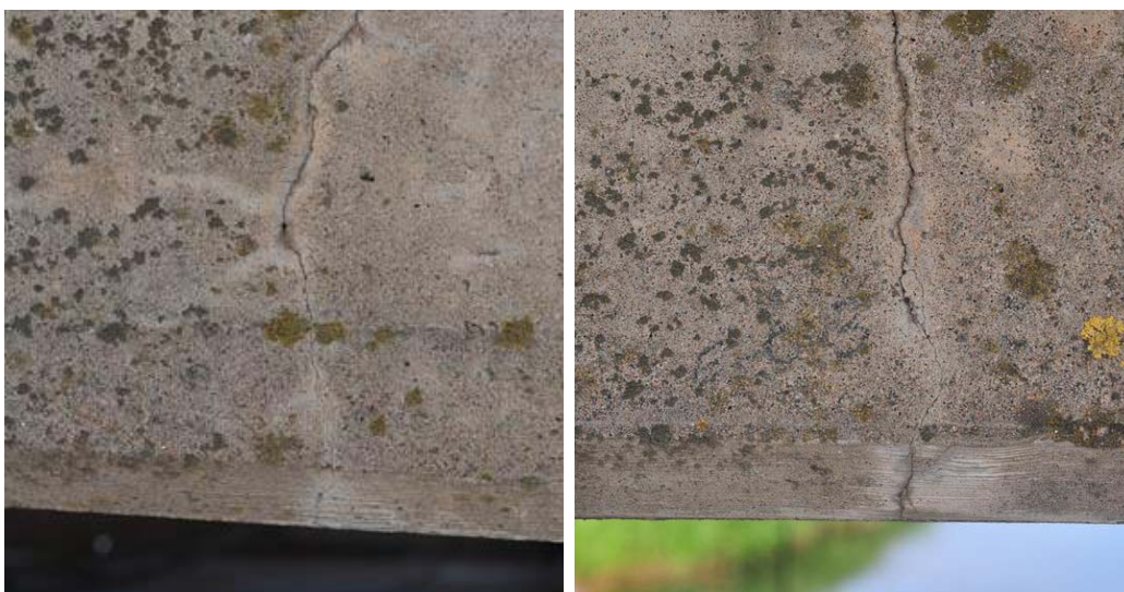
Fig. 3.4 Cracks in the concrete beam at the mid span of the bridge.
