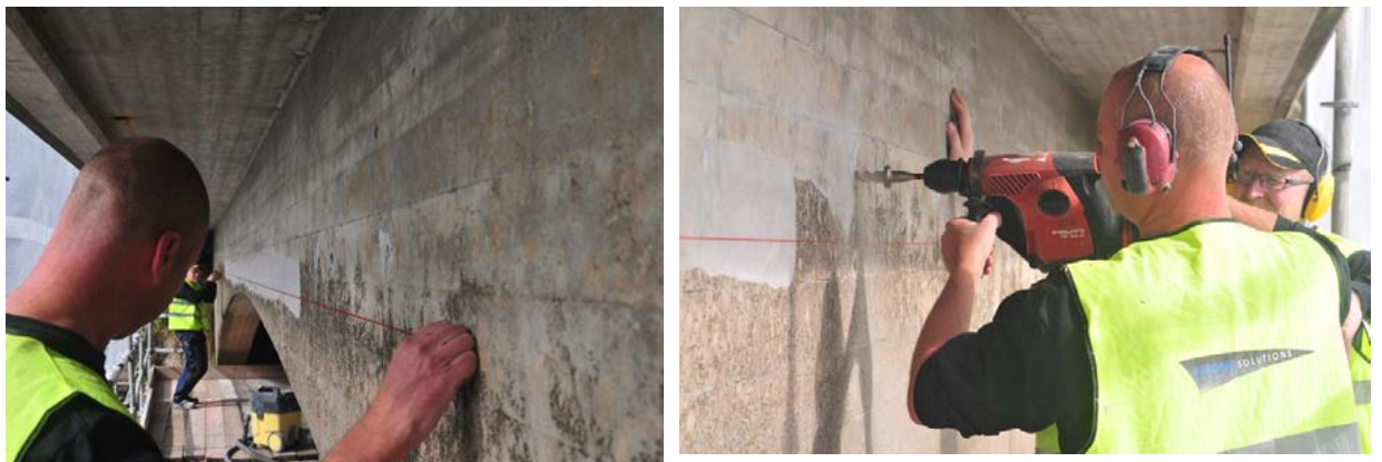
Fig. 5.3 Marking the location of the laminate on the beam (left) and drilling the holes to install Hilti® bolts to fasten temporary steel anchors (right).
